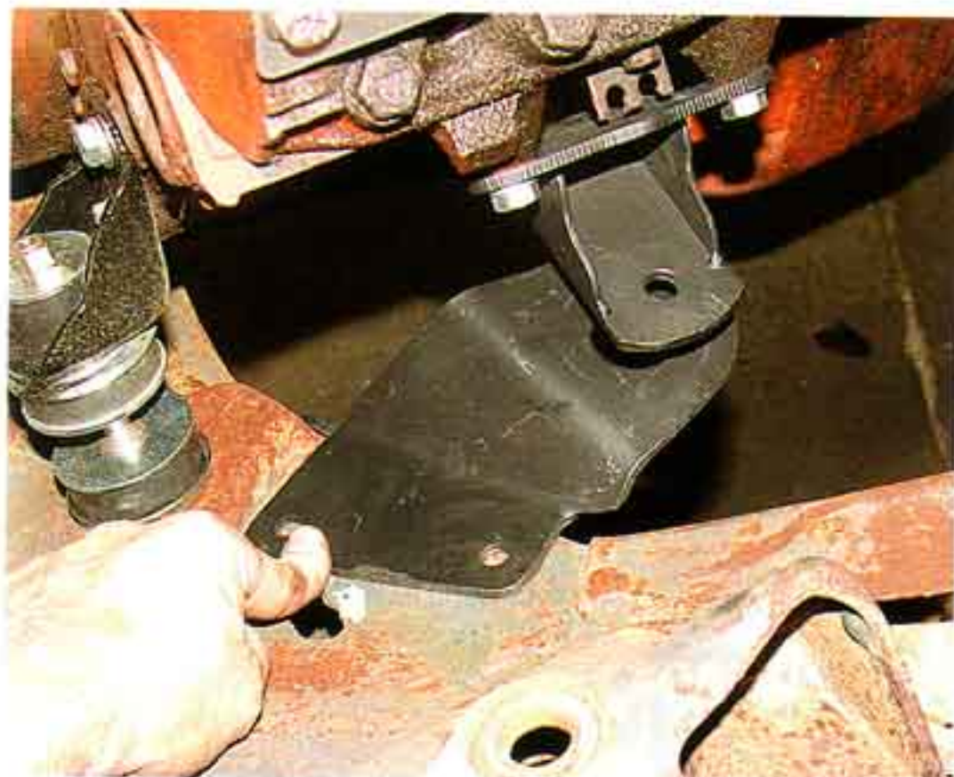
Photo #3: The lower bracket bolts to the top and rear of the original front engine crossmember. The bracket is designed to be bolted in, but may be welded in if you wish.
