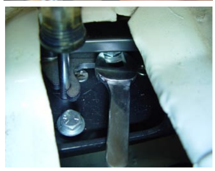
Photo ABO-11a: Shows the procedure with the unit installed and the intercostal sheet metal obscuring access to the Motor Spindle and Spindle Nut.
